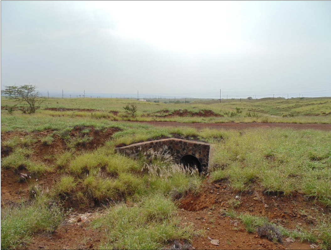
Figure 7. Lālāmilo survey area, culvert beneath the existing access road, view to the west.
